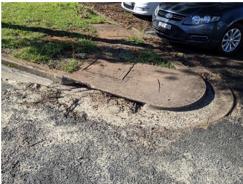
Heavily silted carpark drainage inlets
